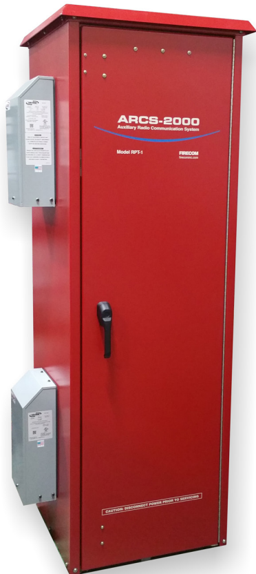
RPT-1 Repeater Cabinet (RAU)
